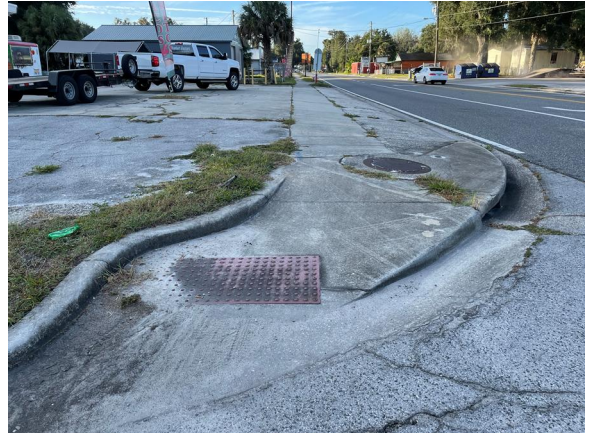
Photograph 26: Existing southern curb ramp at the intersection of SR 471 and NE 4 th Avenue
