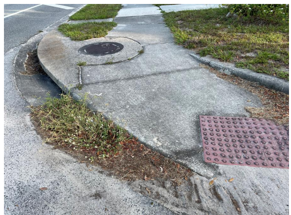
Photograph 24: Existing northern curb ramp at the intersection of SR 471 and NE 2 nd Avenue
