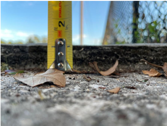
Photograph 27: Gap between sidewalk slabs in front of Webster Elementary School
