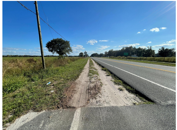
Photograph 28: Visible tire marks extending beyond northbound right-turn lane at southern entrance to Webster Elementary School
