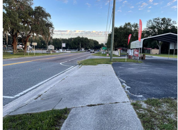
Photograph 8: SR 471—facing north at end of sidewalk on eastern side of corridor
