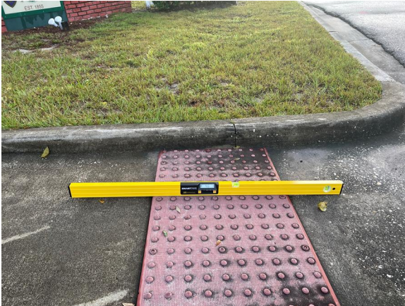
Photograph 7: Grade of northern curb ramp at intersection of SR 471 and eastbound Central Avenue
