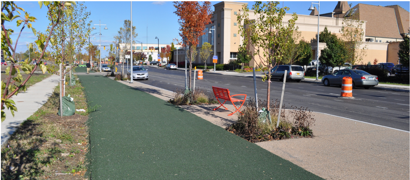
Newly constructed protected bike lane with street trees. Photo courtesy of Stantec and City of Rochester.
