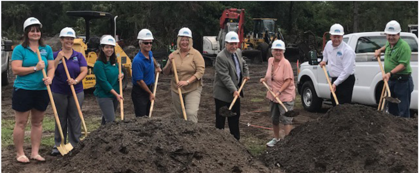
Dale Street Trail Groundbreaking (Edgewater) 1st Groundbreaking for a SUN Trail project
